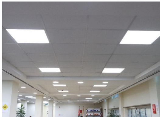
Figure 9: LED lighting in library.
