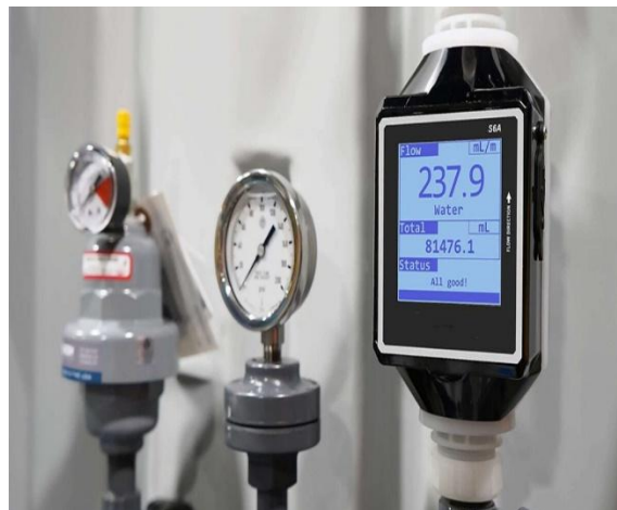
Figure 26: Water flow meters.
