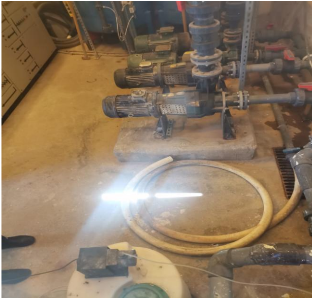
Filtration and chlorination system
