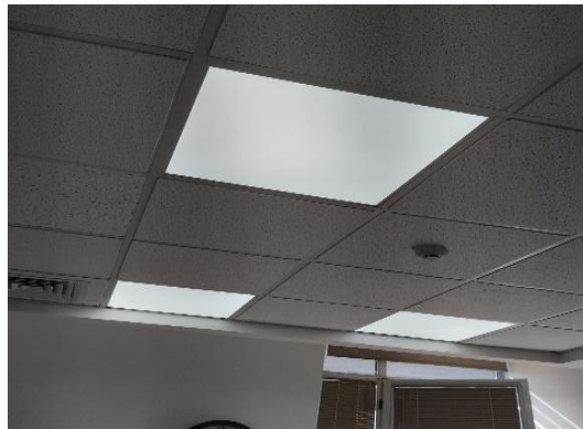
Figure 8: LED lighting in classrooms.
