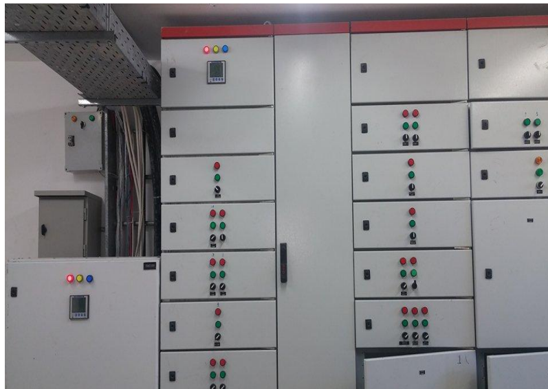
Figure 17: Building (C) BMS.
