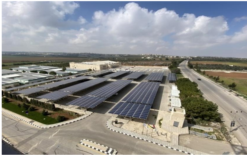
Figure 11: PV System car park.
