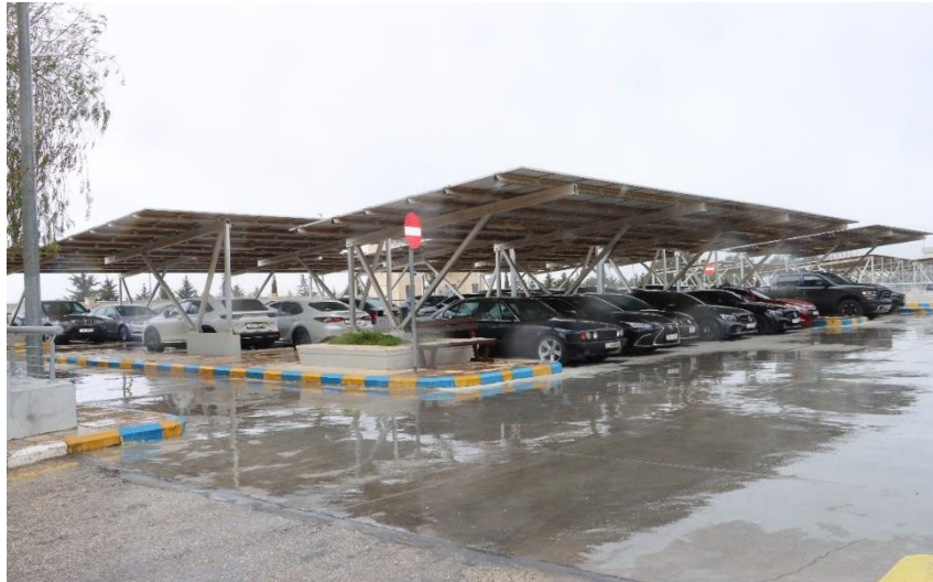
Figure 13: PV car park.
