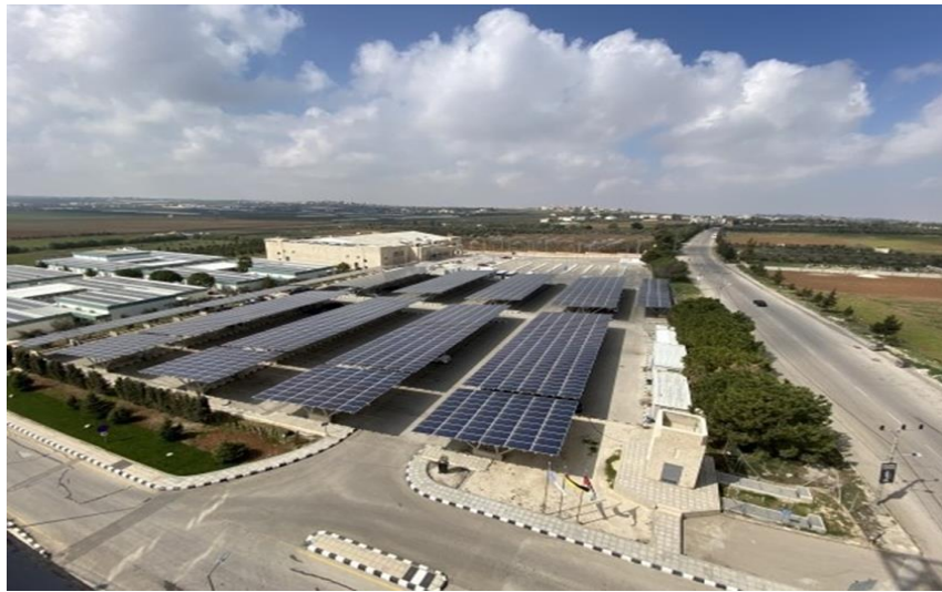
Figure 11: PV System car park.
