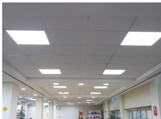
Figure 9: LED lighting in library.
