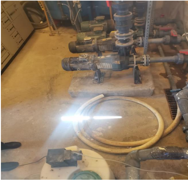
Filtration and chlorination system
