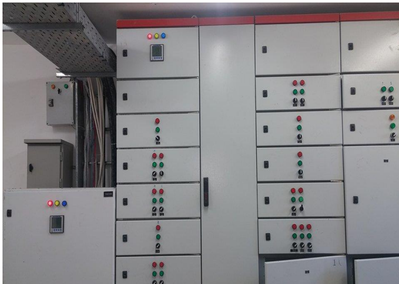
Figure 17: Building (C) BMS.
