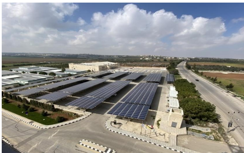
Figure 11: PV System car park.
