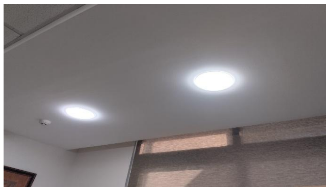
Figure 10: LED lighting in offices.
