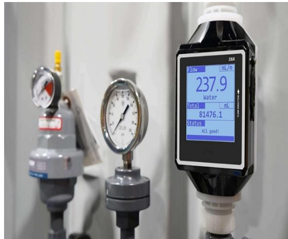
Figure 22: Water flow meters.
