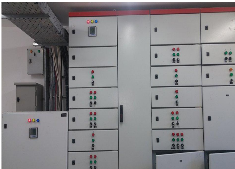
Figure 16: Building (C) BMS.
