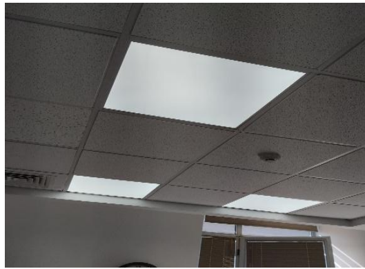
Figure 8: LED lighting in classrooms.
