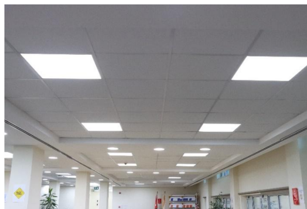
Figure 9: LED lighting in library.
