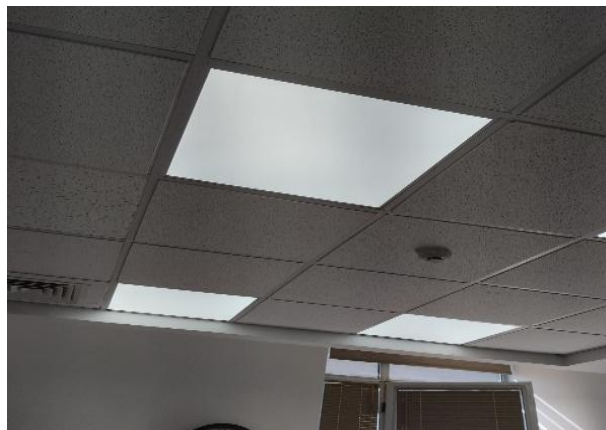
Figure 8: LED lighting in classrooms.
