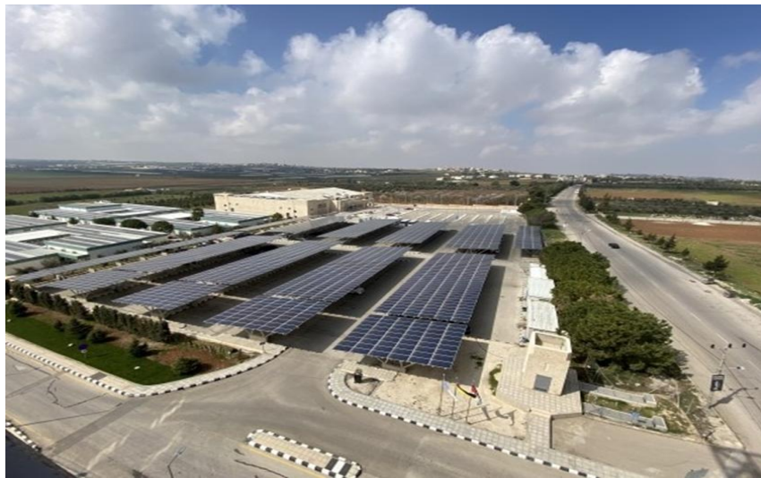
Figure 11: PV System car park.
